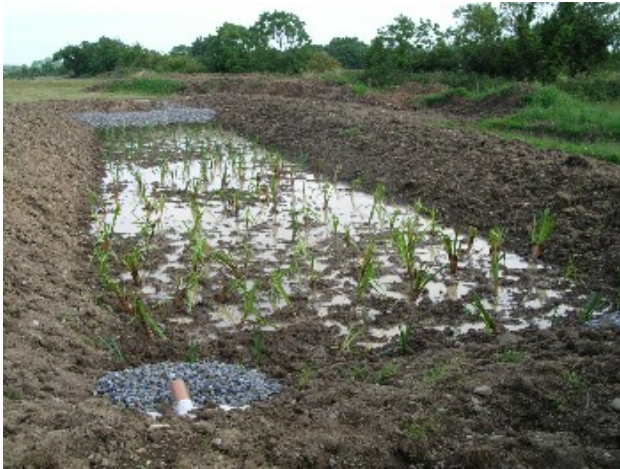
Newly planted wetland system for single dwelling, filled with clean water for planting and plant establishment.
